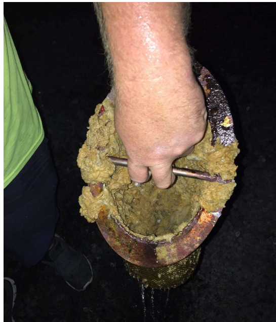
Sponge fouled pipeline at KPLG tenant's farm at HOST Park. (photo credit BOM)
