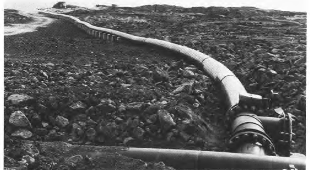
The newly installed 18-inch diameter emergency back-up pipeline snakes across the lava towards the sea. This pipeline will deliver 3000 gpm of deep cold seawater to NELH projects.
