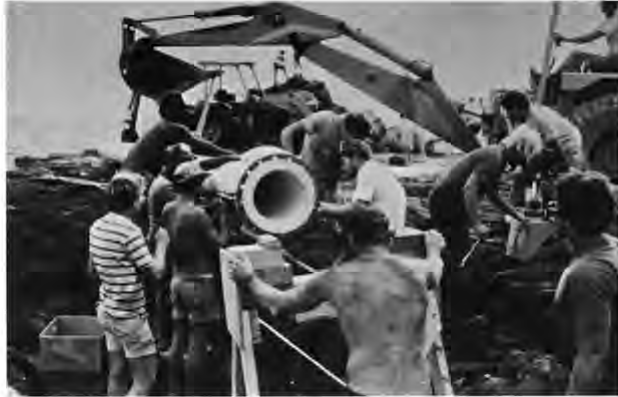
All hands at work on the installation of a Hawaiian Abalone Farms deep seawater pipeline, August 1986.
