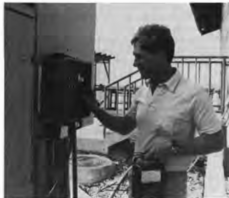
Bud Placek checks the cold water pump panel.
