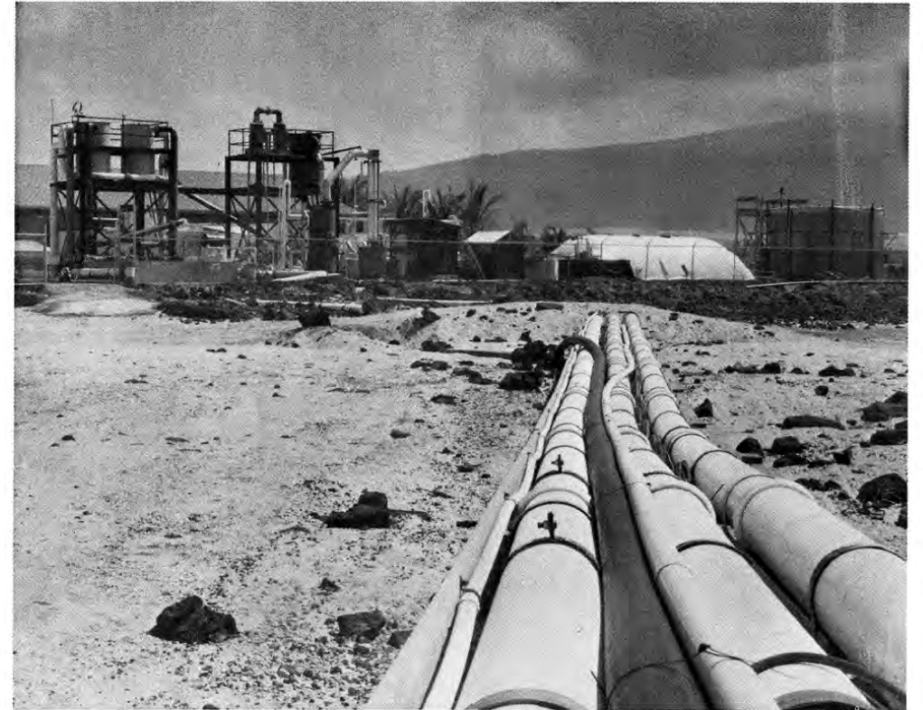
Seawater pipelines with laboratory in background.
