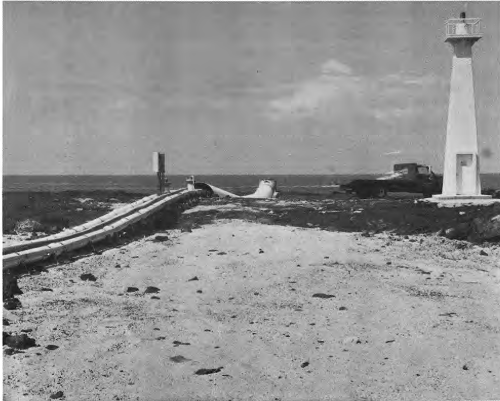
Onshore section of seawater pipelines. Note protective cover extending from the lighthouse to shore.
