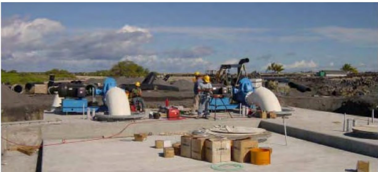
Work on the new deep seawater pump intake plumbing at the 55-inch diameter pipeline pump station in December 2003.
