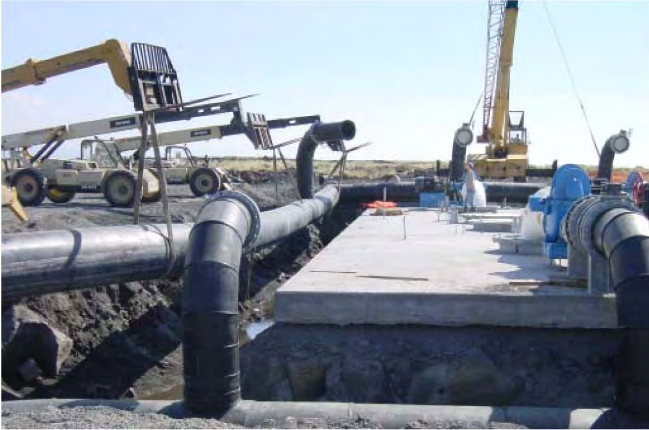
In one of the final stages of installation in December 2003, three forklifts and a crane prepare to synchronize lifting of the entire surface seawater discharge manifold plumbing into a trench at NELHA's new 55-inch pipeline pump station in HOST Park.
