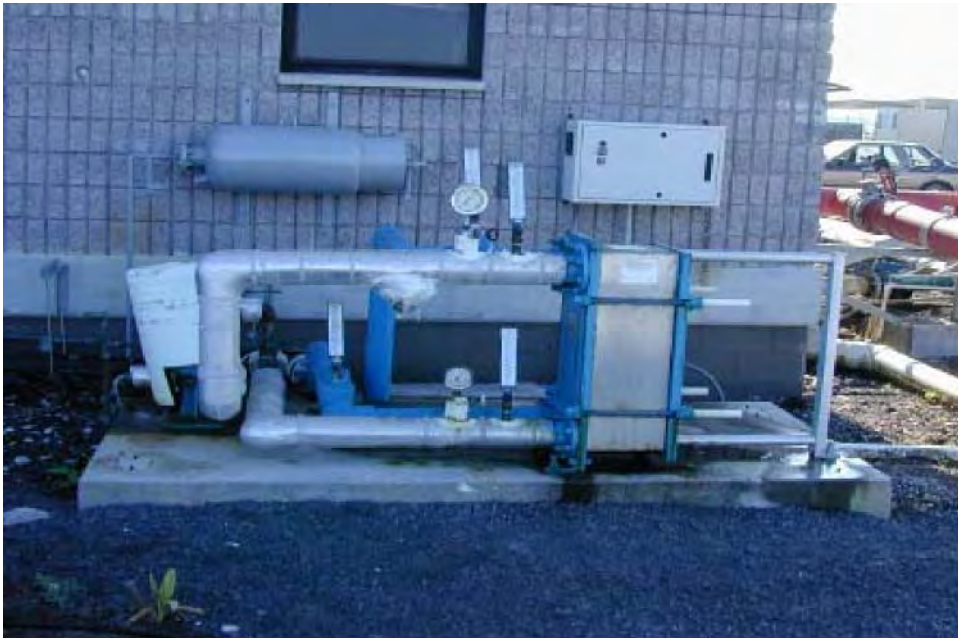
A simple heat exchanger is at the heart of deep seawater-based cooling in the Research Compound.
