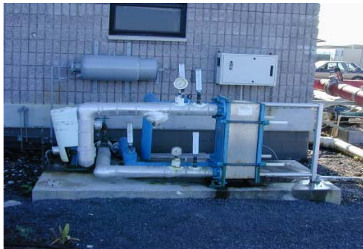
A simple heat exchanger is at the heart of deep seawater-based cooling in the Research Compound.
