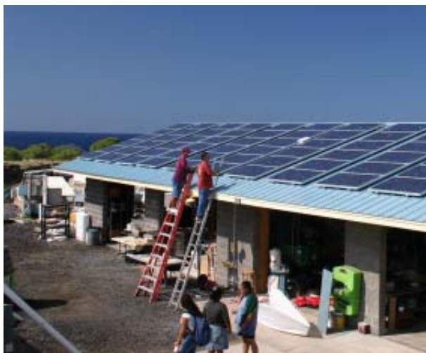
WHEA students and adult colleagues work collaboratively on final stages of installation of new photovoltaic panels at the public charter school's NELHA site.
