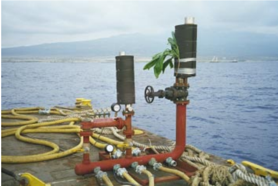
Shipboard view of work deck during the deployment of the 55-inch pipelines during FY 02.
