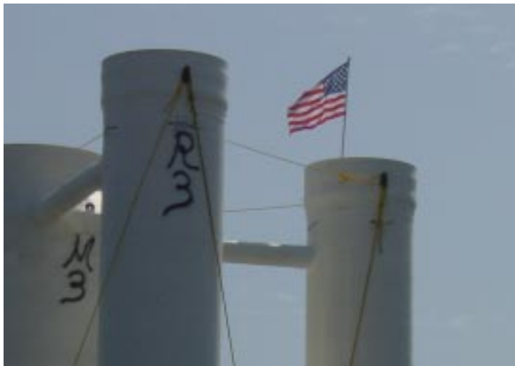
A view of an American flag posted by the work crew on the pump station canisters prior to installation at the HOST Park work site.
