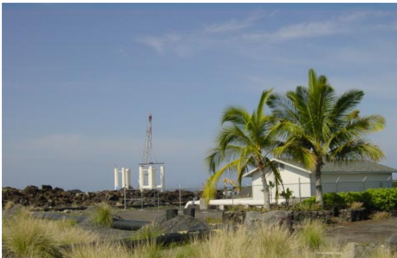
Specially designed, 40-ft. tall white fiberglass reinforced plastic canisters loom in the background south of the HOST Park Booster Pump Station. A crane is lifting one of them into the sump where it will be installed to house the pumps for the new 55-inch pipeline delivery system.
