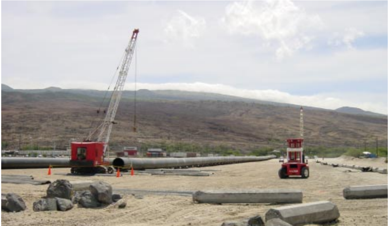
A staging area at Kawaihae Harbor was prepared for the critical pipeline assembly process to fuse the individual pipe sections into 1,000 foot lengths, to later be joined at sea into the final lengths needed for the dual pipeline system.
