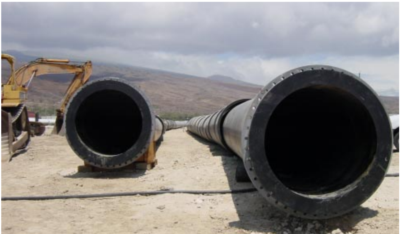
The massive size of the 55-inch pipelines is apparent in this view of the pipelines next to some heavy equipment. The pipes are made of high density polyethylene (HDPE), manufactured on the mainland U.S. and shipped by barge to Hawaii.
