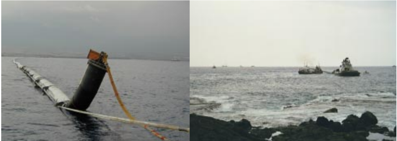
LEFT: The intake end of the deep seawater pipeline floats on the ocean offshore of NELHA's Keahole Point properties while the pipe is being positioned in the critical moments before sinking. RIGHT: Tugboats and other vessels which assisted in the complex process to install the new 55-inch pipeline system.
