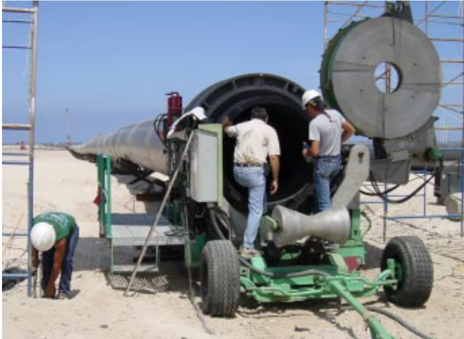
The HDPE pipe sections for the 55-inch pipeline were heat fused using a special fusing apparatus, shown here in this photo. The fuse is said to be stronger than the pipe itself.
