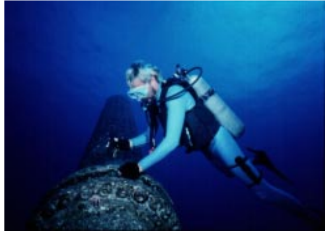
A professional diver works on a pipeline in waters at Keahole Point during early years of NELHA's development
