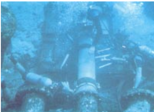
Underwater pumps present maintenance challenges.
