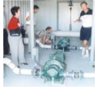
Pump station interior view.
