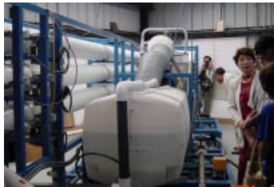
NELHA tenant HDMWPP installed 150-ton reverse osmosis equipment to desalinate deep seawater for a pre-commercial research project.
