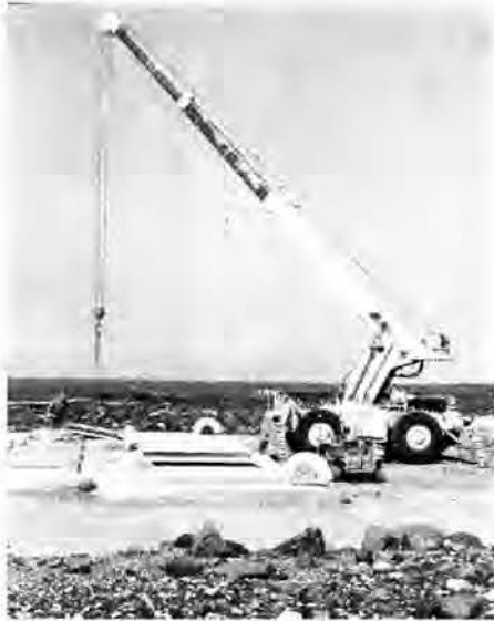
A crane is needed to lift the heavy concrete covers to the NELHA main pump station at Keahole Point.
