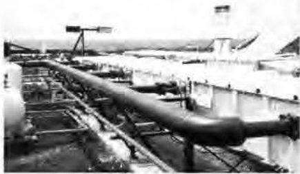
ABOVE: Joe Clarkson of PICHTR explains the workings of NELHA's CC-OTEC experimental plant to a visitor. BELOW: The CC-OTEC flat plate heat exchangers are the focus of testing for this phase of the research process.
