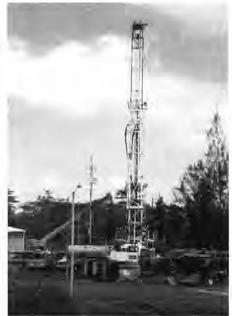
Drill rig looms over the PGF facility site during the plug and abandon procedures for the HGP-A well.
