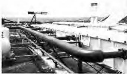
ABOVE: Joe Clarkson of PICHTR explains the workings of NELHA's CC-OTEC experimental plant to a visitor. BELOW: The CC-OTEC flat plate heat exchangers are the focus of testing for this phase of the research process.
