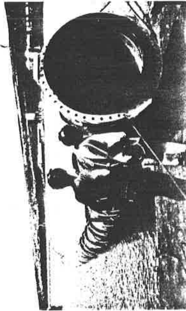
Fig. 6-2. VIEW OF THE 48-INCH CMP AT KAWAIIHAE HARBOR, DURING ATTEMPTED DEPLOYMENT OPERATIONS IN SEPTEMBER-OCTOBER 1993
