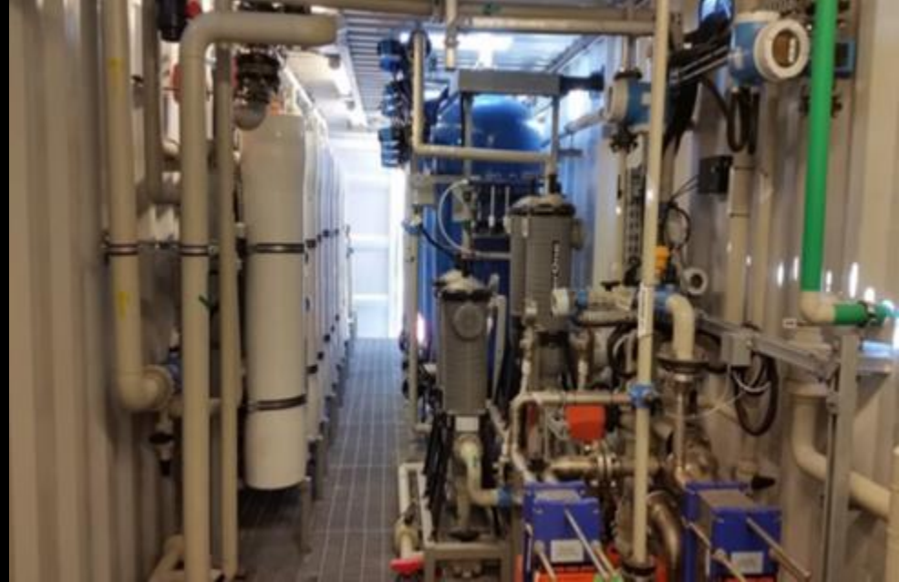
FO membranes, Pre-treatment and Heat recovery HX
