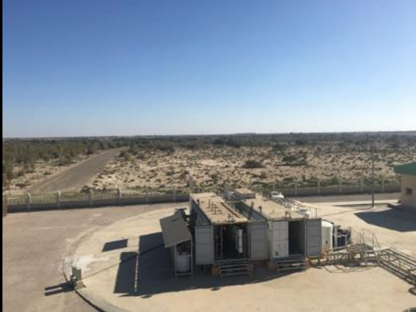
Masdar 2 container 50m3/day Pilot (Outside Dubai)
