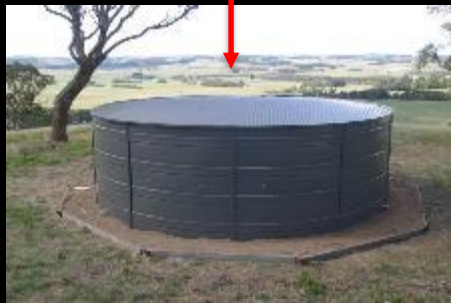
Energy Storage Tank
