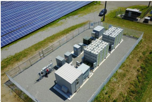
Eos Energy Storage
