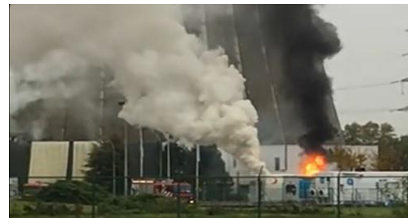
In Nov 2017, this lithium battery with state-of-the-art fire protection technology failed during commissioning, resulting in release of toxic fumes, closing freeways and evacuating citizens
