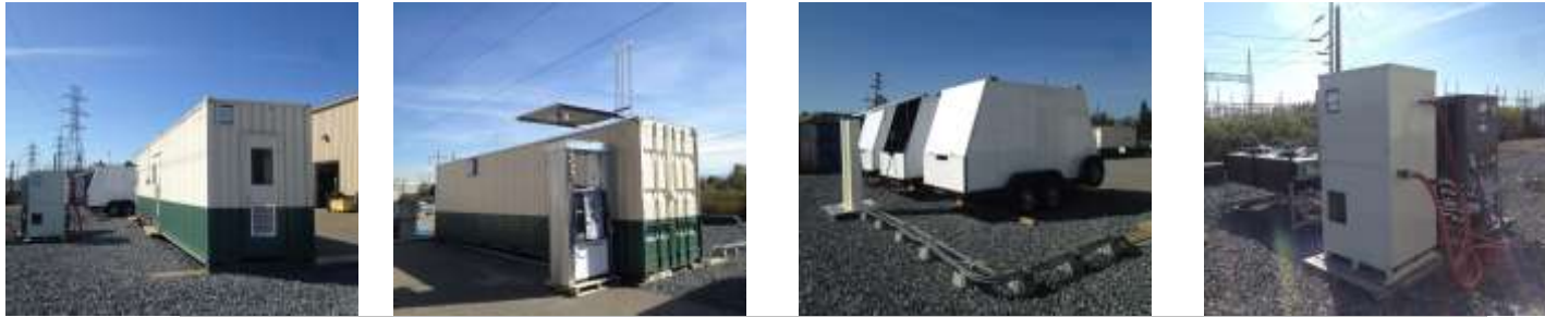
Equipment under test at Powertech
