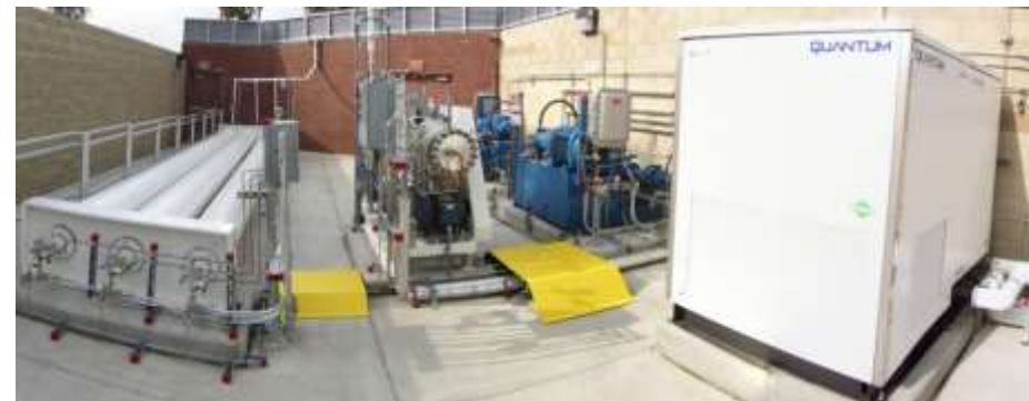
CSULA: PV-electrolysis-based hydrogen station
