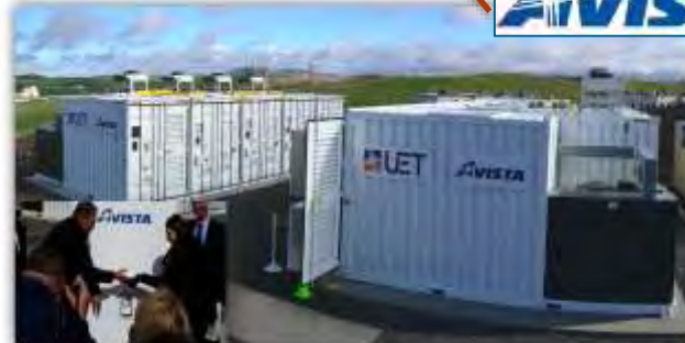
1 MW / 3.2 MWh UET vanadium-flow battery – Pullman, WA
