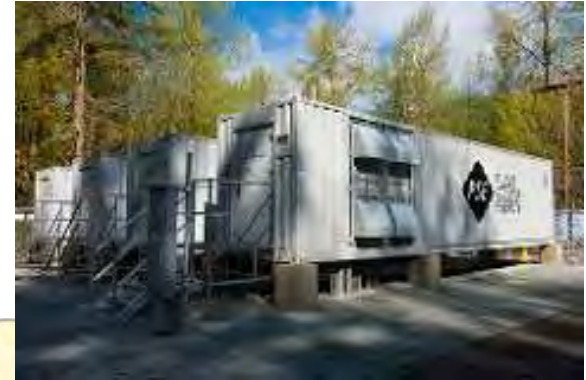
2 MW / 4.4 MWh lithium-ion/phosphate battery – Glacier, WA
