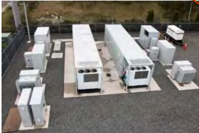
2MW / 1 MWh Li-ion system 2MW, 8.8 MWh UET vanadium-flow- Everett, WA
