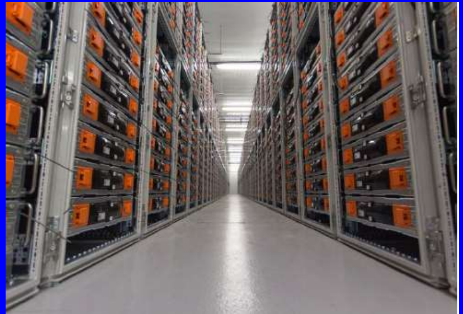
8MW / 32MWh Storage Plant
