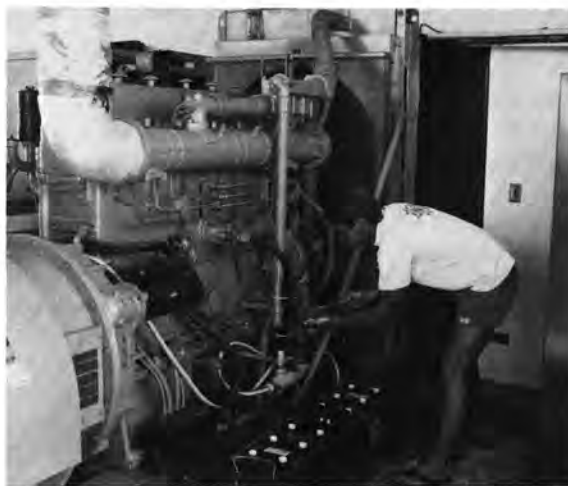
Steve Wilson maintains the backup generators.
