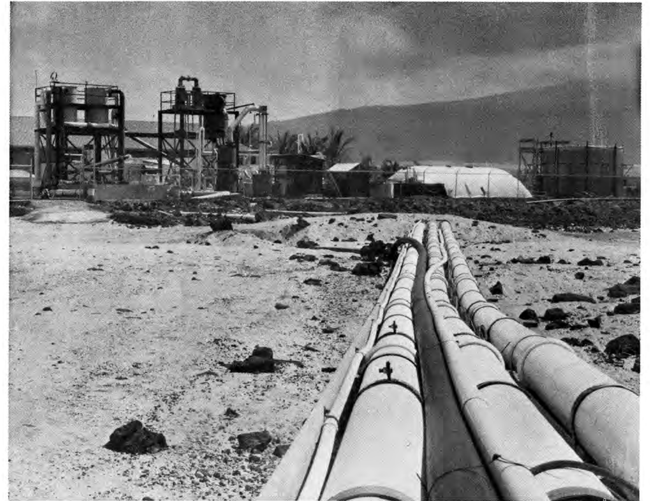
Seawater pipelines with laboratory in background.
