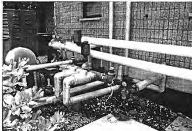
Simple pipes allow cold deep seawater to run into the building air conditioning system at NELHA, saving more than $15,000 per year in taxpayer dollars.
