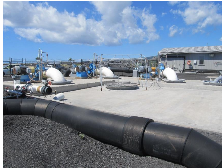
55" DSW pump station
