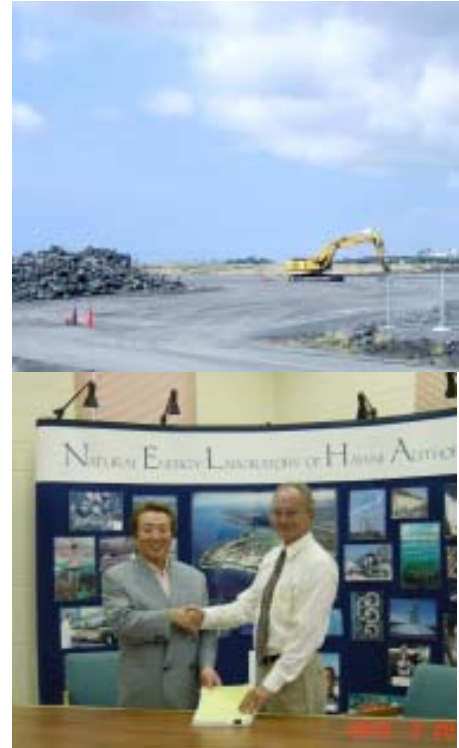
Koyo USA Corp. signed a sublease for a commercial lot at NELHA in February 2002 and was already grading the construction site by June.
